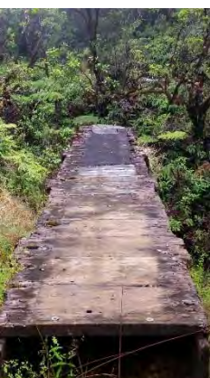
Figure 3: Redwood flume from 1974-1975
