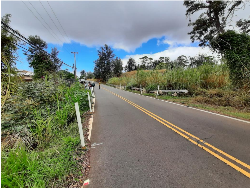
Overtopping damage visible on the downstream guard rail at Lower Kula road
