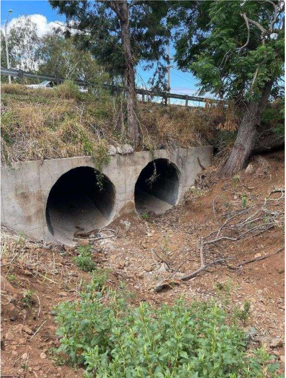
Kula Highway double 10' culvert below Kaluapulani Gulch burn area (recommended upstream clearing and debris removal)
