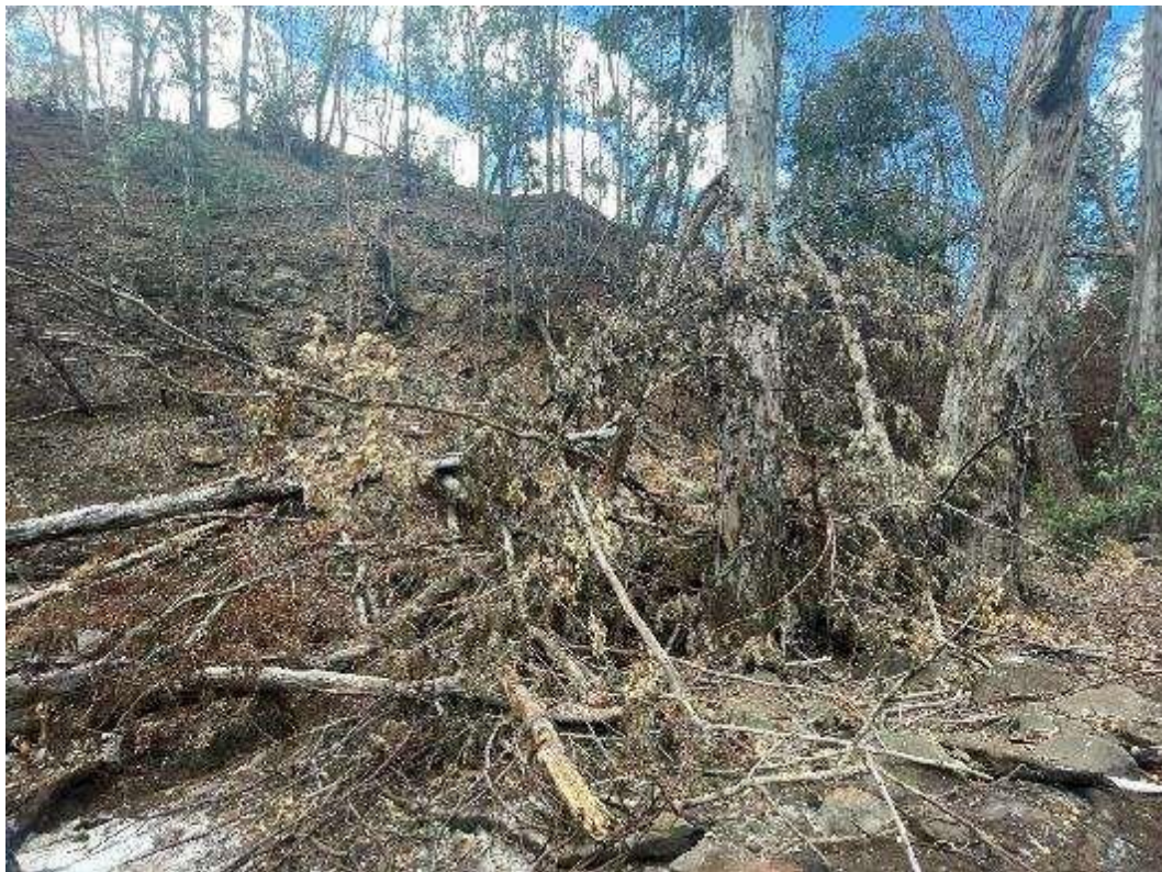
Woody debris in Kaluapulani Gulch (recommend clearing and debris removal)
