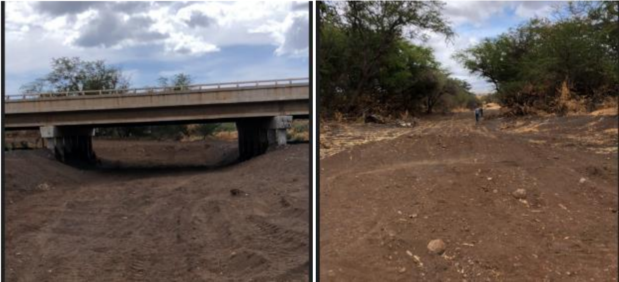
Sediment removal under bridge at Piilani Hwy./Waiakoa Gulch and sediment at Kulanihakoi Gulch)
